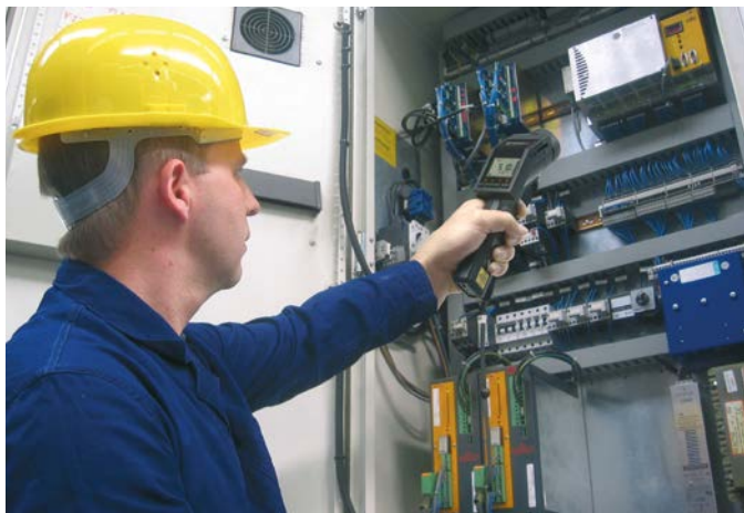
Detailed infrared temperature measurement of an electric control system using the optris® LS integrated close focus optics for 1 mm ranges
